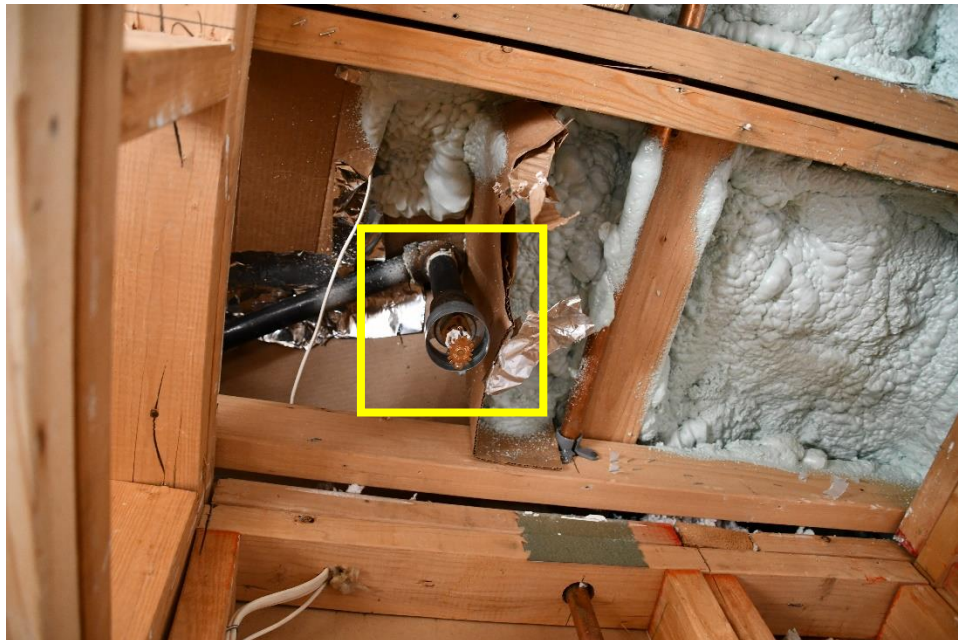
Figure 6. Location of the failed sprinkler head (16020_CBS_1-020).
