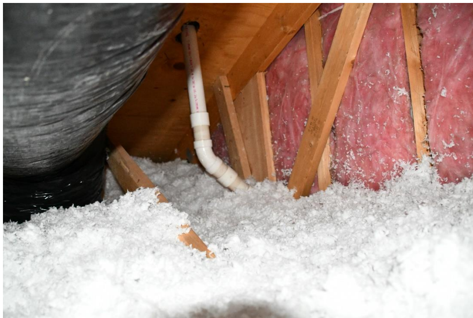
Figure 16. View over the area where the sprinkler branch piping for the subject sprinkler was installed (16020_CBS_1-081).
