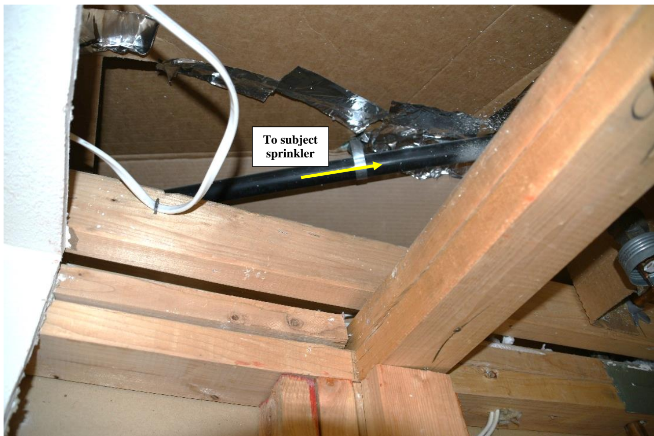
Figure 7. Sprinkler branch for the subject sprinkler head (16020_CBS_1-035).
