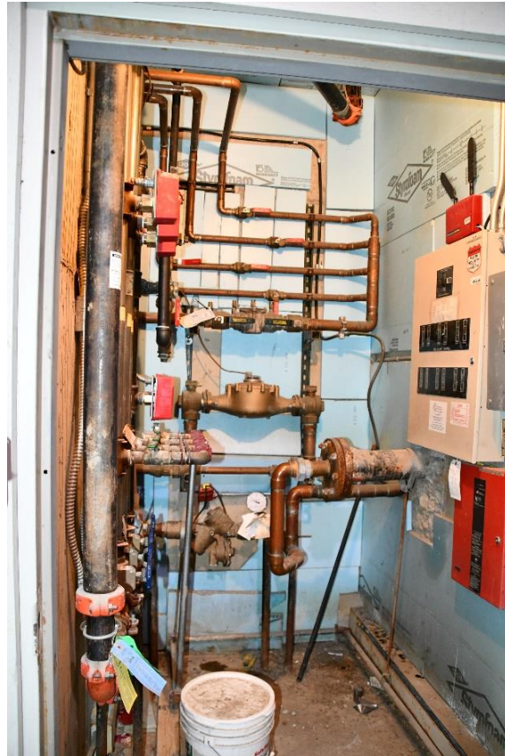
Figure 3. Sprinkler riser room (16020_CBS_1-132).
