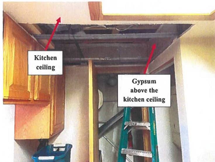
Figure 2. Removed ceiling in kitchen of Unit 304B (15092 CBS 2-006).
