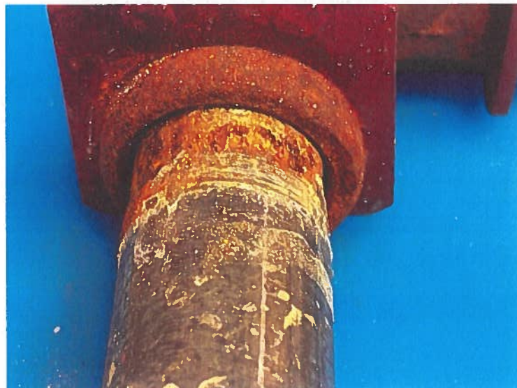
Figure 7. Tubing separating from the elbow fitting (15092 CBS 2-027).
